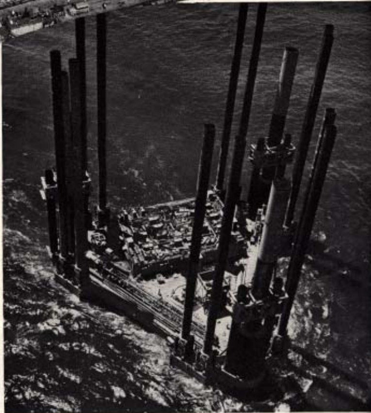
Near-vertical view of tow under way, showing on deck variety of machinery to be used in erecting tower at ultimate location
