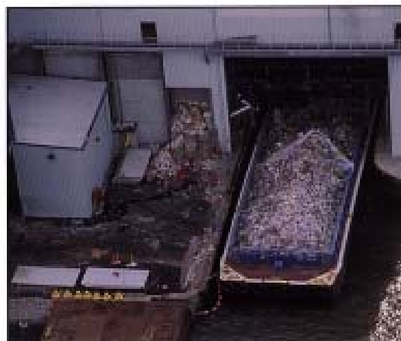
The plant was constructed with a special enclosed barge unloading shed at the dock to prevent polluting the Arthur Kill Waterway.
