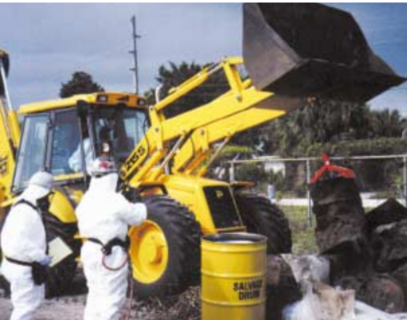
Unknown drum recovery (bottom, left). Steel plant decontamination involving heavy metals and low level radiation (bottom, right).
