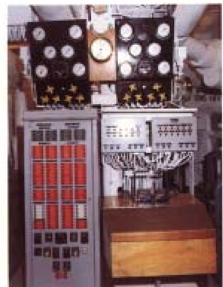
MIRIAM MORAN's engine room control station showing a totally new computer-controlled automation panel designed by Moran's Construction & Repair Department.
