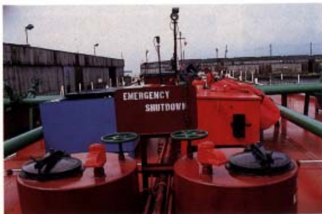
Fire stations, extinguishers, emergency shut off, are all clearly marked on the tank barges. The powder blue colored pollution gear locker in the background stands out.
