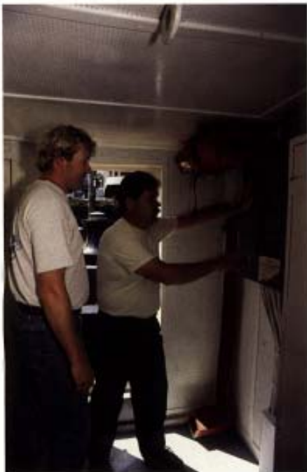
Crew members reviews the electrical panel switches at an onboard training session. Cross-training of the crew is stressed, having deck or engine members know one another duties and equipment.
